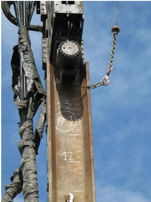
Figure 2.2 Driving of sheet piles using a vibrator attached to the top of the sheet pile web.
