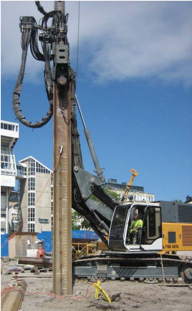
Figure 3.8 Photo of driving equipment and the driving of sheet pile S1 in the Solna tramway field test.
