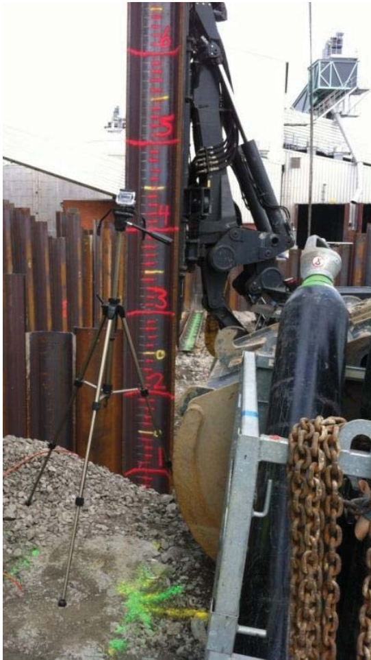
Figure 3.11 Photo of driving equipment and the driving of S1 during the Värta harbour field test.
